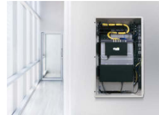
A look inside VWM-PD-4-36K-PW outfitted with C2G cabling, Middle Atlantic Power, and a Luxul switch.
